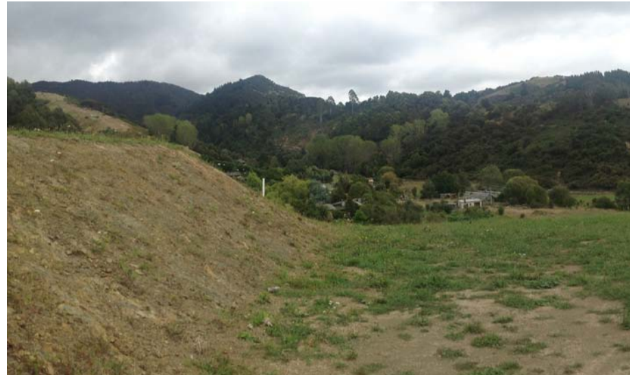
Above: Flattened platforms have been formed along spurs in order to accommodate future residential development.
