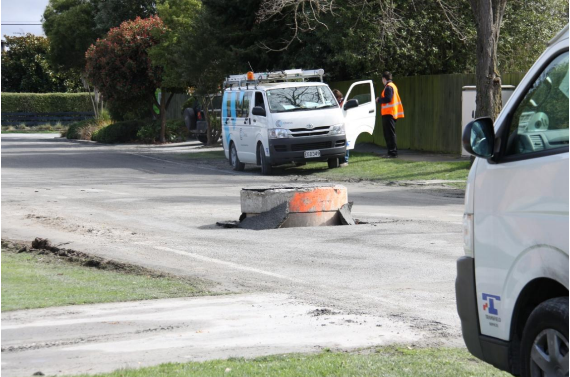
Figure B3: Manhole uplifted due to buoyancy
